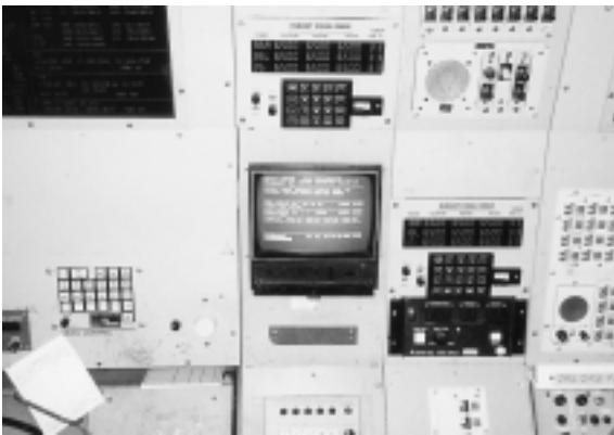
SAIDS-2 needs replacing: it is not Y2K compliant.
