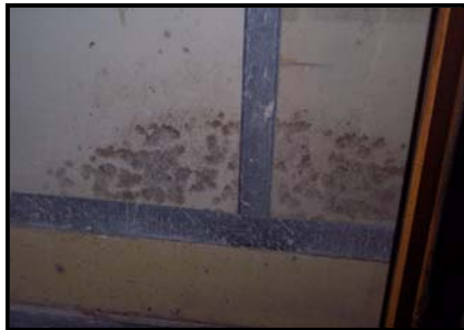
Mold in elevator shaft in Detroit
