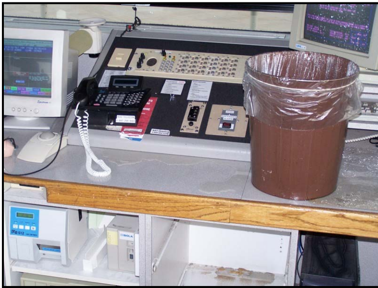
Rainfall leak onto equipment at Grand Rapids, Mich. Tower
