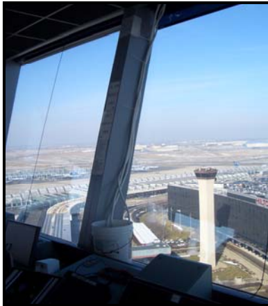
Tower cab at O’Hare using hoses and buckets to capture water leaks
