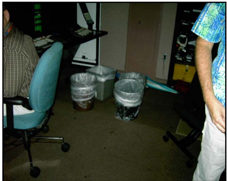
Leaking roof at Atlanta Center
